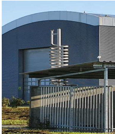
Figure 17 Close up of vent stack at NLR Marknesse
