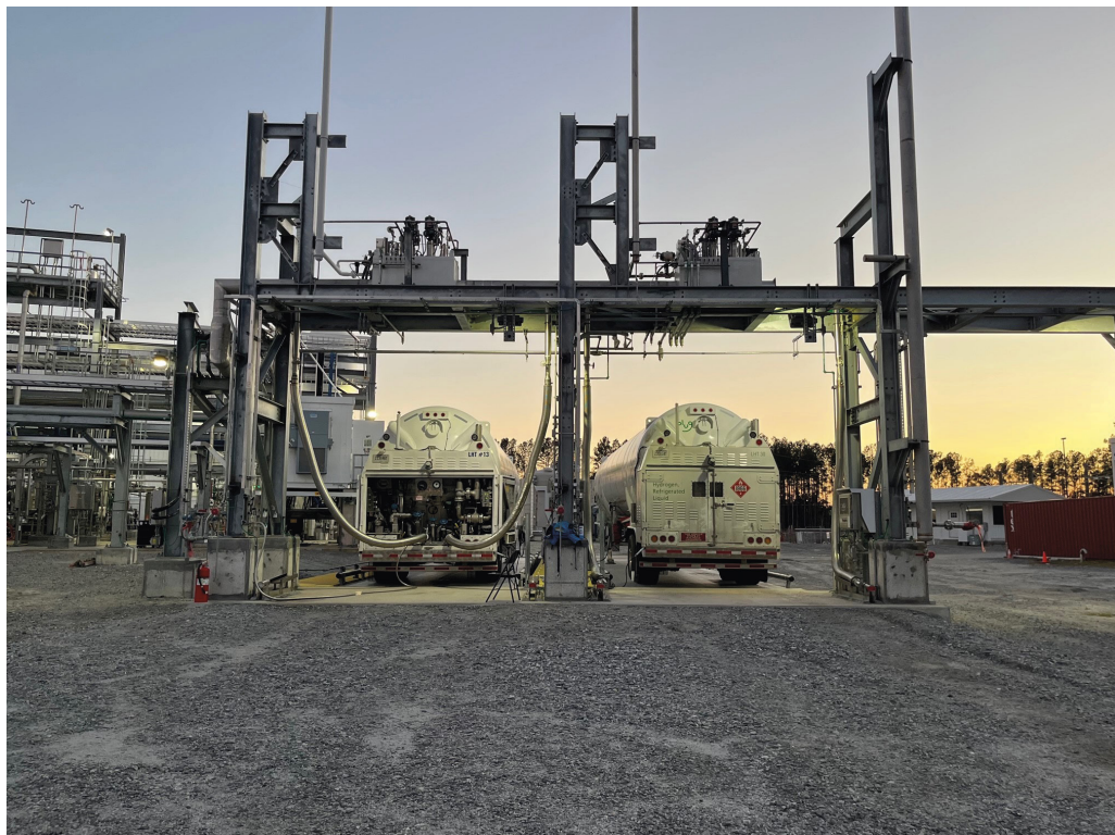
Figure 12 LH 2 loading bays at Plug Power's liquefaction plant in Georgia, USA Source: Plug Power, Inc.
