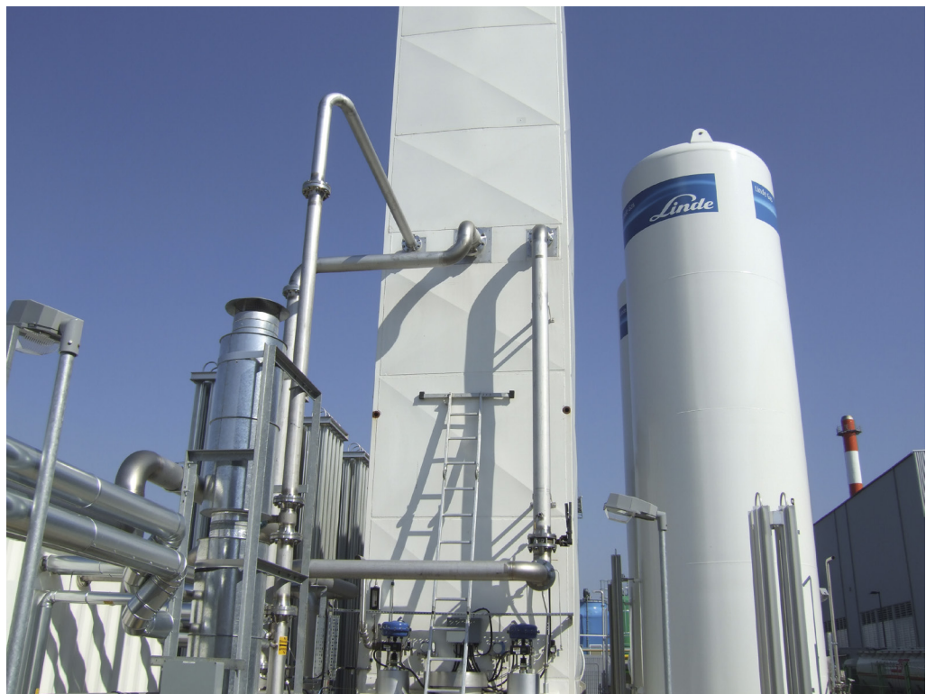
Figure 9 Cryogenic distillation column by Linde as part of an air separation plant Source: Linde
