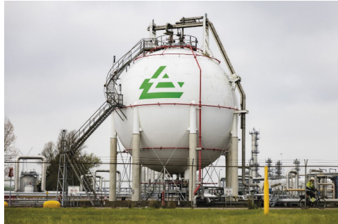
Figure 11 70 t spherical LH 2 storage at Air Products in Rotterdam, The Netherlands Source: Air Products
