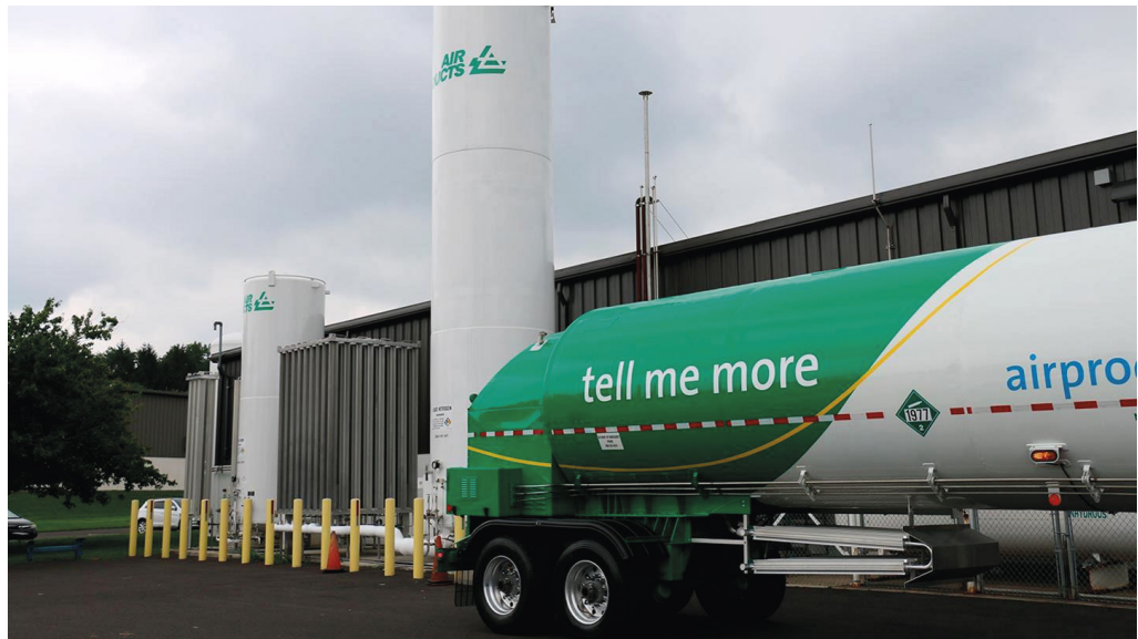
Figure 8 LN 2 tank trailer and fixed storage tank Source: Air Products
