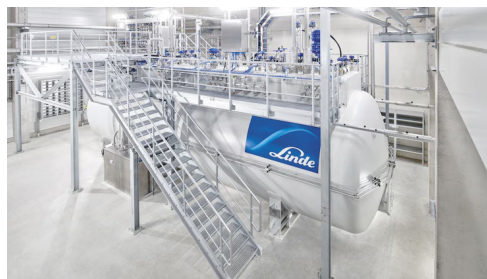
Figure 10 Vacuum hydrogen cold box at Linde's liquefaction plant in Leuna, Germany Source: Linde 87
