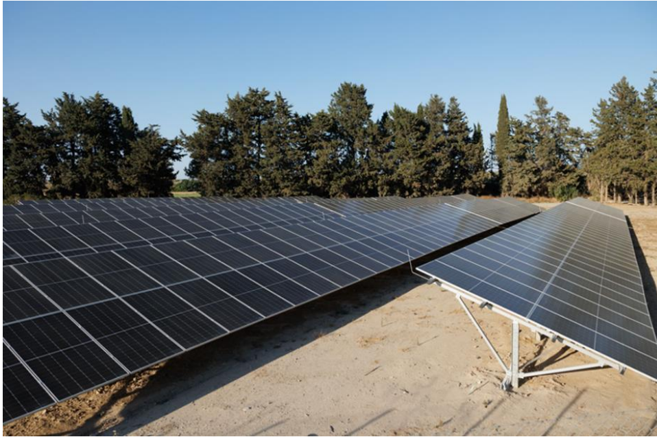
Figure 38, Larnaca Photovoltaic (solar) Park
