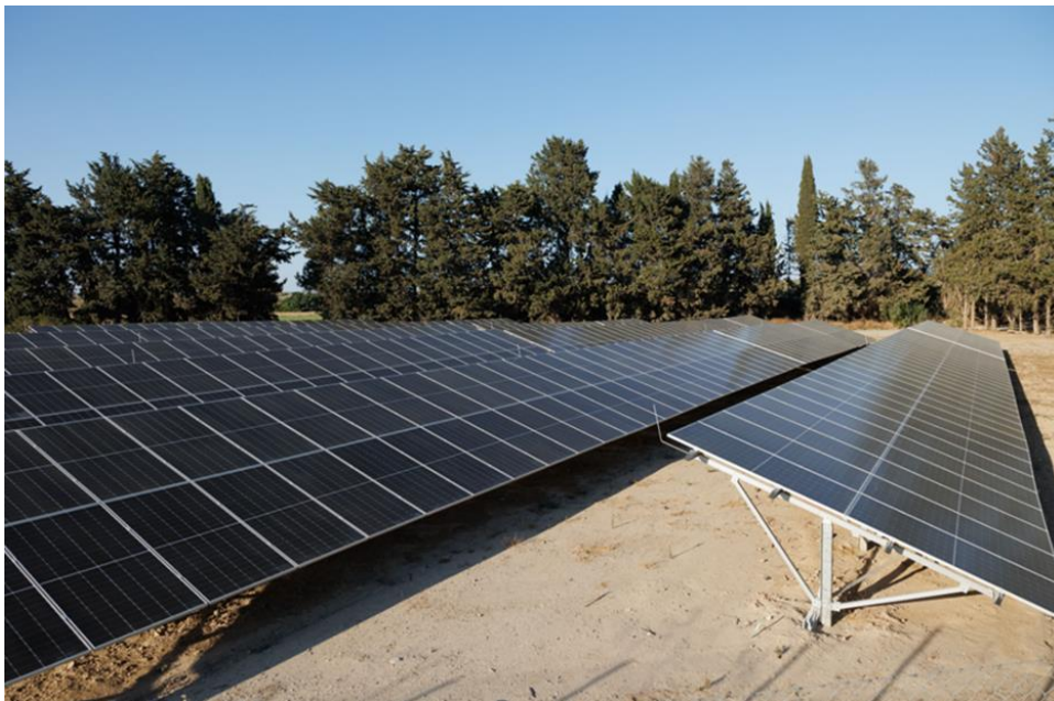
Figure 6.2, Larnaka Photovoltaic (solar) Park
